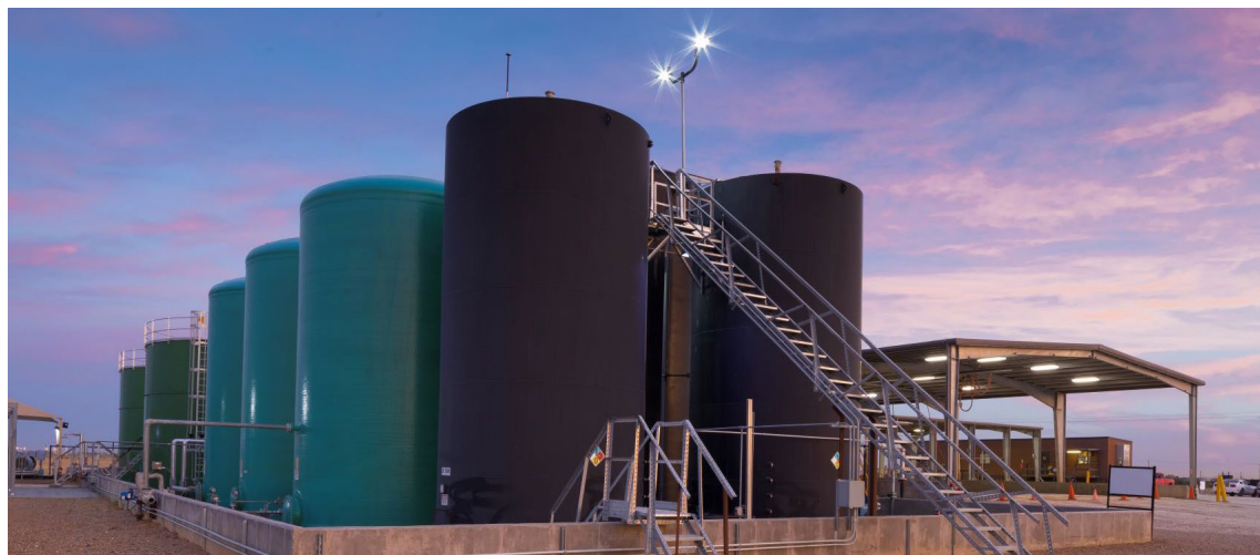
+ Waste injection reduces carbon emitted into the environment and is the environmentally superior solution to land application.
